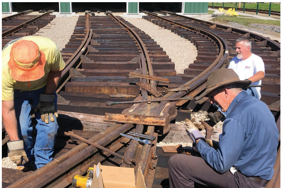
Below: Track crew members work on re-assembling the yard leading to South Boston 2. KO
