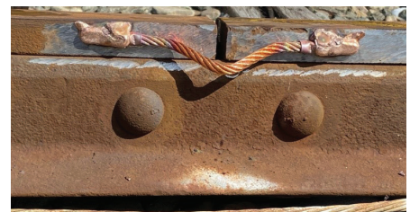
Above: A rail bond welded across a bolted joint.
