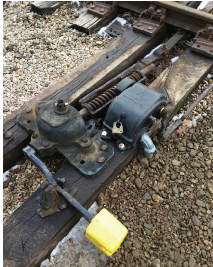
Above: Another view of the circuit controller. DD
