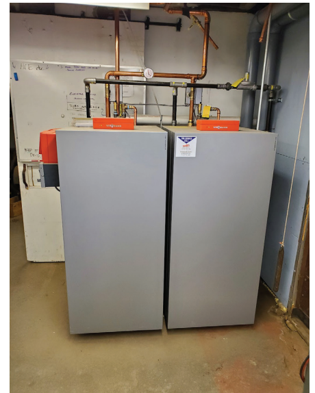
A new heating system in the shop uses less fuel while putting out more heat. DR
