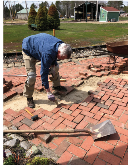
Volunteer Rick Whetstone works on leveling the main brick platform at the Visitors Center. KO
