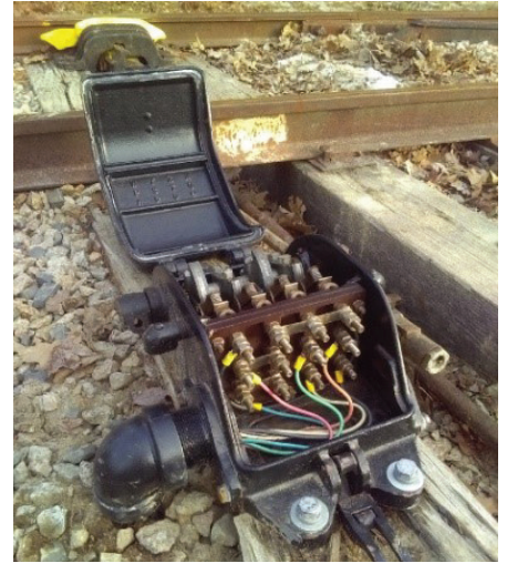
Ground level signal mechanism at the derail. DD
