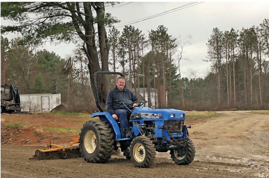
Veteran member Chuck Griffith grades the service road passing the site of the planned bus display. KO
