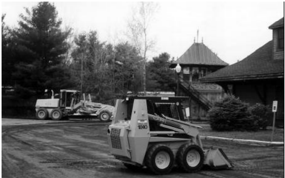
Below: Equipment from Museum corporate member Dayton Sand and Gravel of Dayton, Maine lend a professional touch to resurfacing the roadway and parking area in front of the Visitors Center. PM
