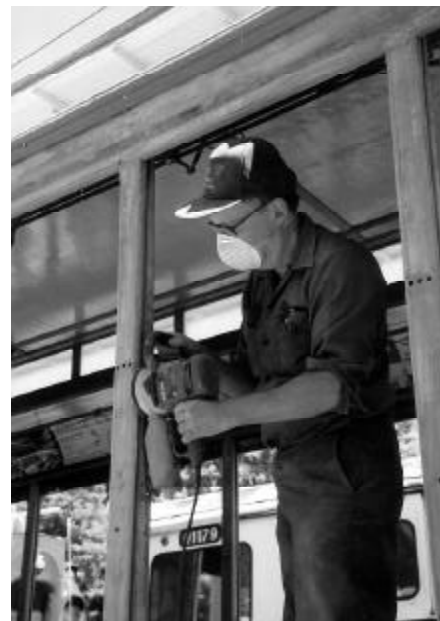
Above: Donations, many from members of the operating department, have made this project possible. Donald Curry power sands a post. DC
