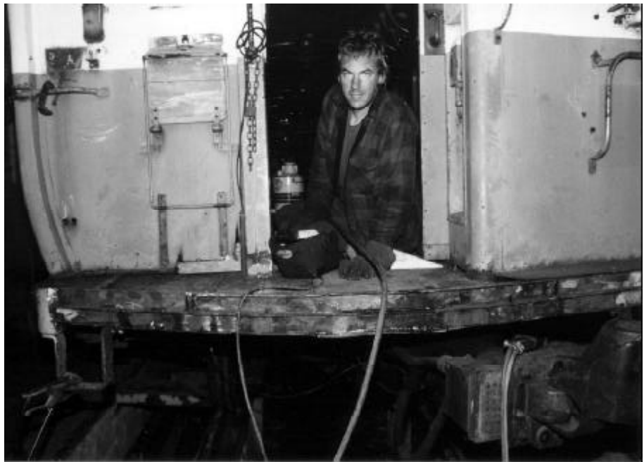
Above: Project sponsor Bill Pollman makes repairs to corroded steel on the end platforms of Boston elevated car 01179. These 1957 cars were built by Pullman in Worcester, MA, and for nearly three decades provided services above the streets of Boston on the Orange Line elevated route. DC
