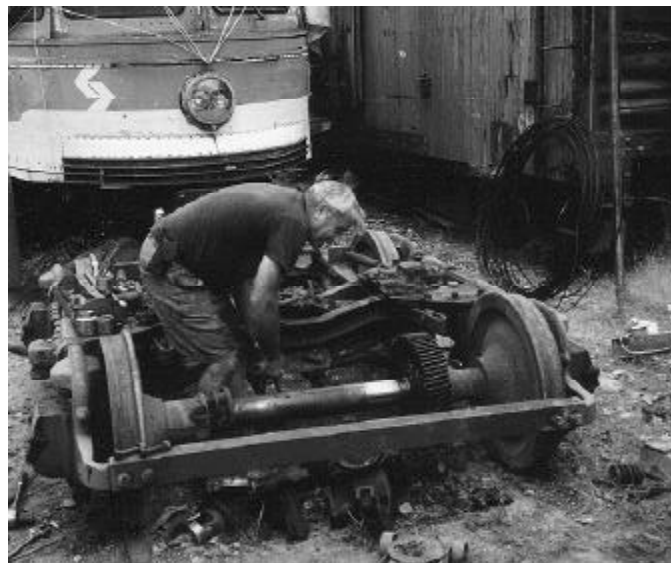
Above: Fred Perry works on disassembling one of 2890's trucks. Toronto track gauge is 2 and 3/8 inches wider than standard, so the wheels and brake rigging require relocation for operation on standard gauge track. FM
