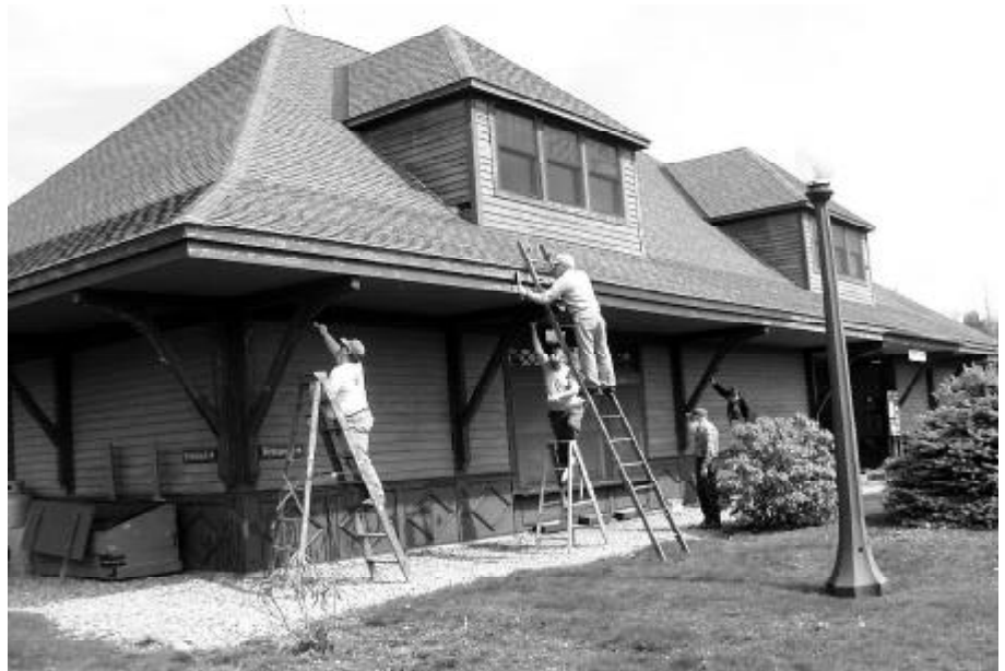
Above: A group of volunteers applies a fresh coat of green and brown stain to the Museum's Visitors Center. The building houses orientation exhibits, ticket sales, the Museum Store, a limited food service, rest rooms, and—on the second floor—the Society's administrative offices. JS
