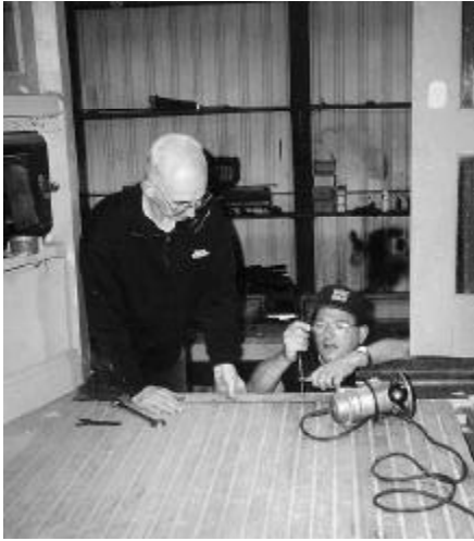
Above: Volunteers Bruce Bardes and Ed Dooks carefully fit one of the wear plates that protects the floor boards and serves as the bottom guide rail for the sliding door on Wheeling 639. FM
