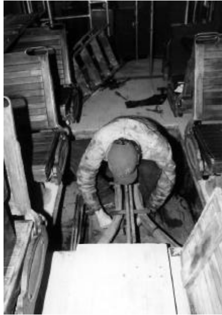
Above: Chris Perry undertakes a periodic motor inspection on Dallas 434. "Motor traps," removable sections of floor, provide ready access. DC
