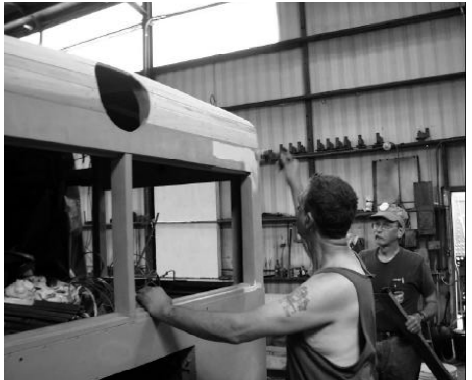
Below: An enthusiastically supported volunteer project is the rebuilding of Boston & Maine Railroad inspection car 500 to preserve the car and for use by the Museum's track department. Here Gary Jenness applies primer on newly installed wood as project sponsor Ben Yuscavitch looks on. JS
