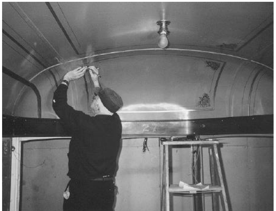
Below: Ken Haselton very carefully applies the floral pattern to the corners of the striping in Cleveland 1227. Ken made decals of the pattern based on surviving samples of the original ceiling. The complete headlining of the car has been replaced, including the very complex curved end sections. FM
