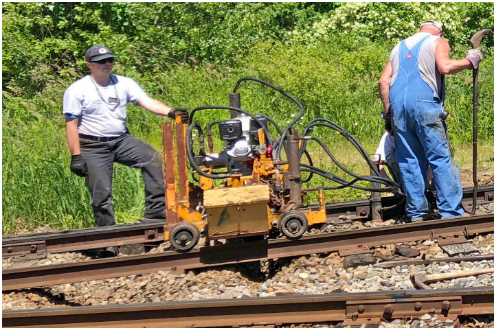
Above: John Petillo works with other members of the track crew to replace deteriorated ties on the Visitors Center loop. JS
