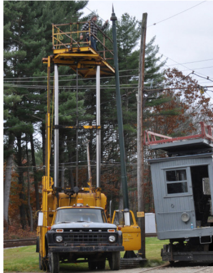
Above: Claremont line car No. 4 is back in service, shown here participating in a bracket arm replacement with a rubber tired equivalent. TS
