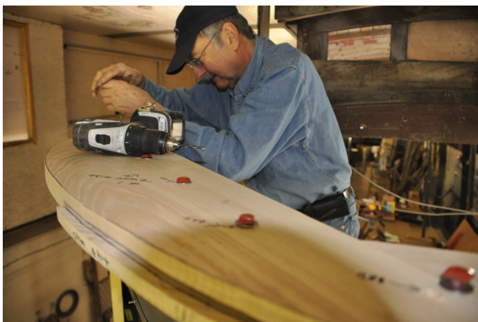
Above: Volunteer John Mercurio screws down the flat plate that connects the curved roof bonnet to the front platform framing on Boston Elevated Railway Center-Entrance No. 6131, a long-term restoration project. DC
