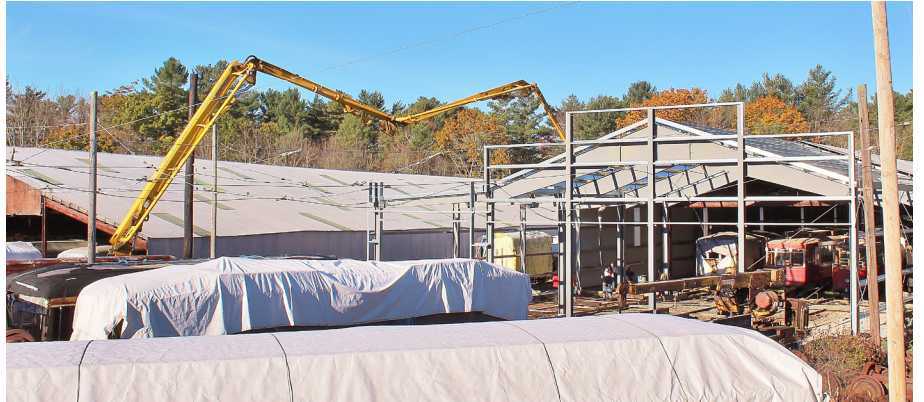
Top Left: Excavation for the front foundation of the Fairview extension. Top Right: Concrete is being poured for the rear concrete pad. Above: A very long concrete pump pours the front concrete pad. TS
