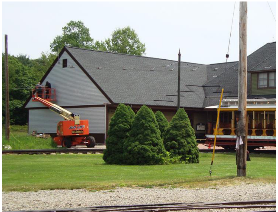
Above: The Visitors Center got new siding and paint during summer 2018 with help by members Tom Tello and Jim Mackell, shown here putting finishing touches from the platform of a boom-lift. KO
