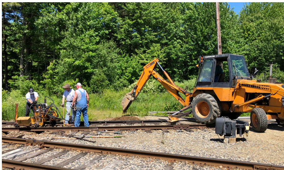
Below: Seashore's track crew hard at work replacing deteriorated ties on the Visitors Center loop. JS
