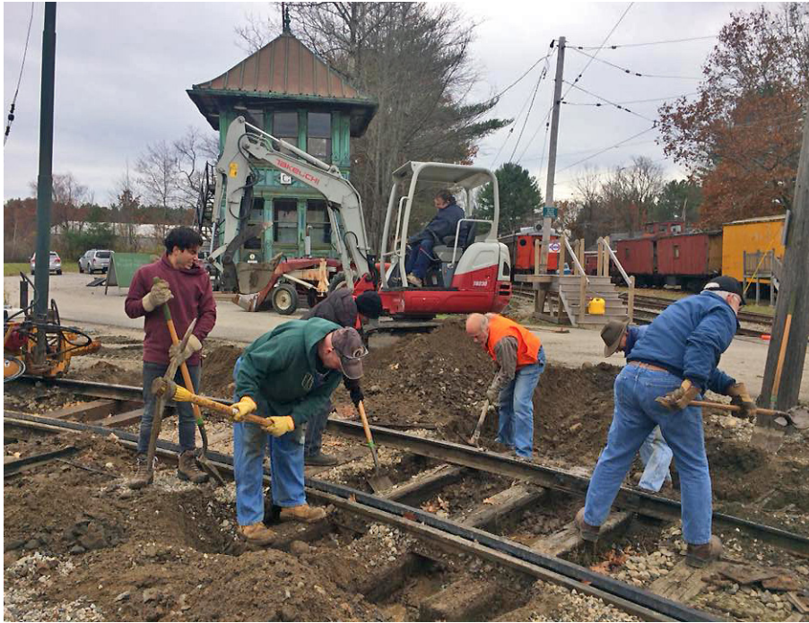
Above: The track department is hard at work replacing deteriorated ties in the Visitors Center loop during a work weekend in November 2018. KO
