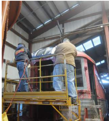
Above: Eric Gilman and Tom Tello work on framing to support the protective wooden mat on the end of the roof of Chicago, North Shore & Milwaukee high speed interurban 755. DC
