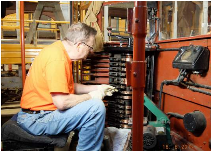
Above: The high voltage K controllers used in most conventional streetcars require constant attention as breaking the current flows to the motors causes internal arcing. Here Ed Dooks adjusts the contact fingers in Boston Type 5 5821. DC
