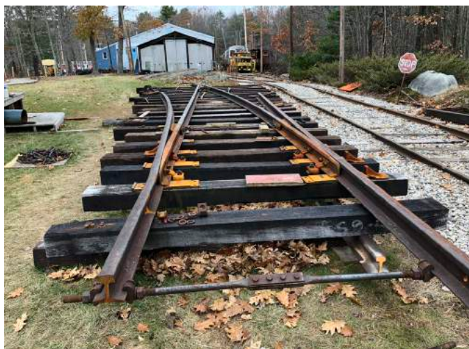
Right: A new No. 4 switch is assembled next to the Shop lead. It will replace a badly worn switch (once part of the Atlantic Shore Line network in Sanford) just visible in front of the yellow track machine at the top center. When complete the switch will be lifted in place by a crane. JS
