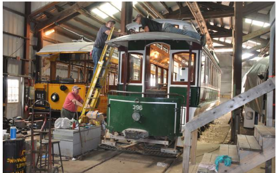
Above: The program to upgrade Boston Elevated Railway 25-foot box car 396 continues on a time-available basis. Here Dick Avy, Jim Mackell, and John Melanson work on renewing the car's roof canvas. A century ago Boston had a fleet of over 1,200 of these cars, of which this is the only survivor. DC
