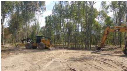
Above: Some of the heavy equipment used by the timber harvesters shown in a newly cleared staging area. PM
