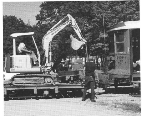
Above: Track crew members Peter Wilson and Ben Yuscavitch prepare to do some drainage ditch maintenance using a rented backhoe. JS
