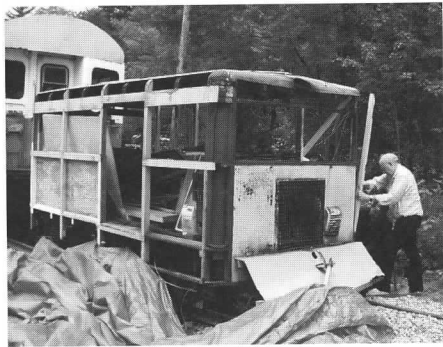
Above: Volunteers from the Museum's track crew are thoroughly rebuilding B&M inspection car 500. Here a new cornerpost is fitted. JS
