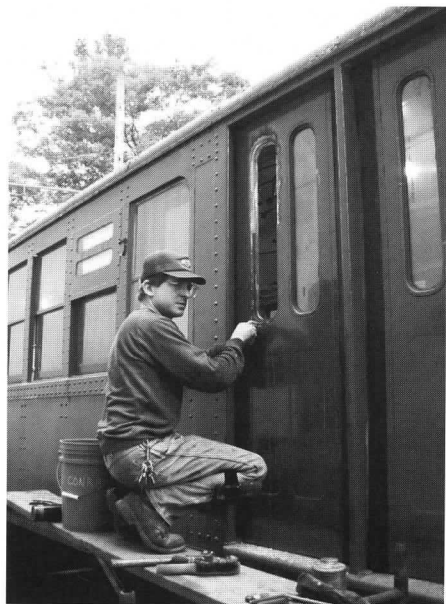
Above: Conrad Misesk, sponsor of Philadelphia-Camden subway car 1023, repairs a door window, as the exterior nears completion. JS
