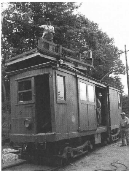
Above: A volunteer crew uses Claremont, NH line car No. 4 to undertake some maintenance on the overhead wire in the authentic manner. JS
