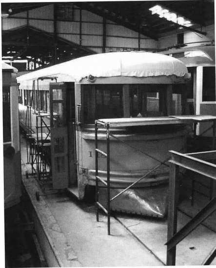
Above: Cedar Rapids and Iowa City interurban 118 received new roof canvas during the year. JS
