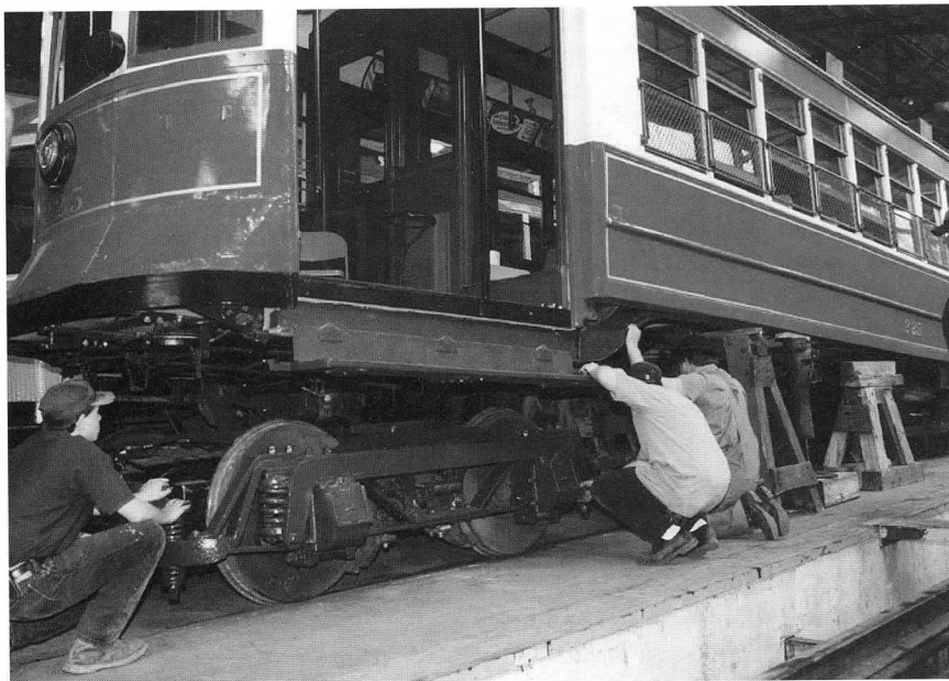
Above: One of the final steps in the restoration process: After thorough overhaul and reassembly, Chicago 225’s second truck is rolled under the car. Shop crew members John Arico, Charlie Hammond, and Mike Simonds carefully check clearances and alignment. DC
