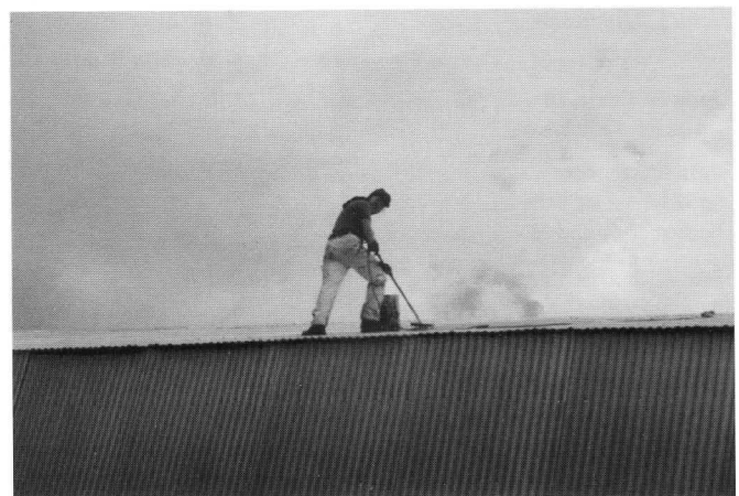
Above: Volunteer Conrad Misk applying sealant to the roof of Highwood Carhouse. This step helps prolong the life of the aluminum sheathing, though the roof surface will ultimately need replacement. FM
