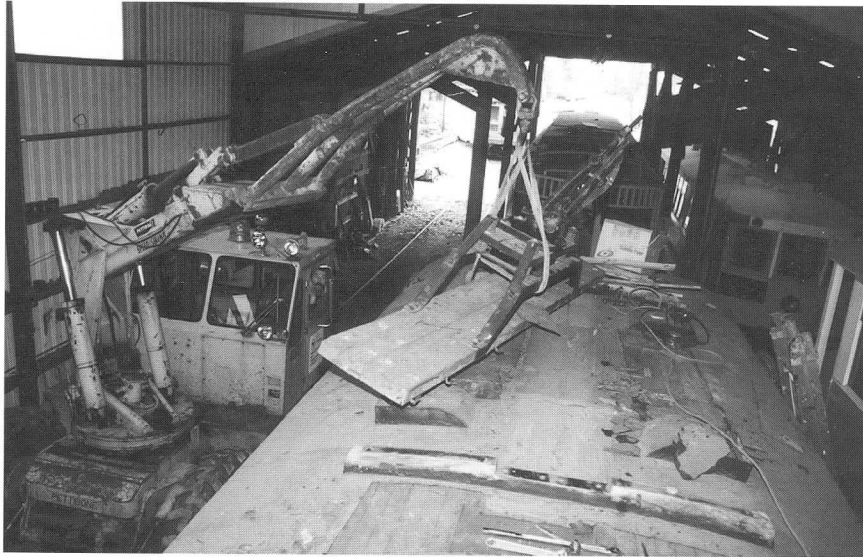
Above: Shop crew member Gary Jenness carefully maneuvers the Pettibone Speedswing to lift the trolley boards from the roof of No. 118. Roof repairs require removal of all boards and hardware, then canvas, followed by inspection and patching of the underlying boards. DC
