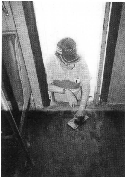
Above: Hervey Lesch smooths a freshly patched section of the floor of Philadelphia-Camden subway "Bridge Car" 1018. DC
