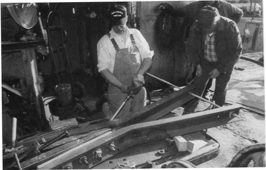
Above: Track Superintendent Peter Wilson, helped by Dick Avy, uses a torch to heat the rail to modify the angle of the track frog for installation at Arundel Station. This complex task was necessary as no suitable frog could be found to replace a temporary frog installed years ago. DC
