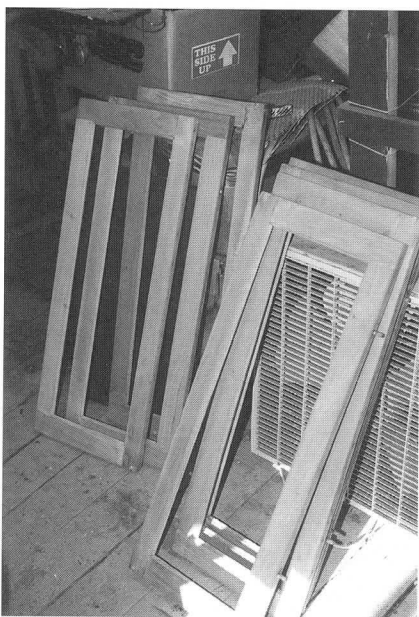
Above: Upper window sash frames for 1160 after thorough stripping and repair. RS
