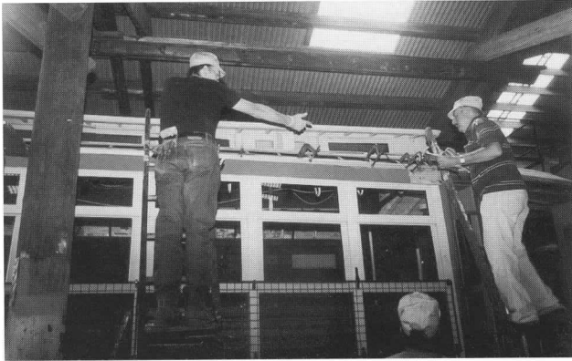
Above: Ben Yuscavitch and Dick White repair a deteriorated section of roof on Eastern Mass. Street Railway No. 4387. DC
