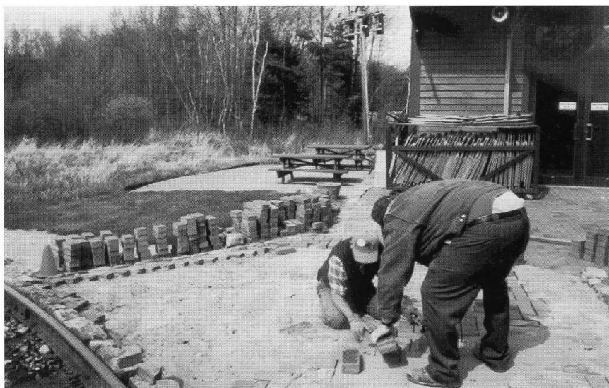
Above: Dan Heffner and Dick Avy work on resetting the brick platform at the Visitors Center, after winter freeze and thaw cycles had led to an uneven base for the bricks. DC
