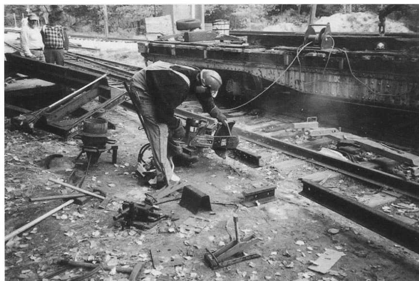
Above: Track Superintendent Peter Wilson uses a gasoline-powered abrasive saw to cut a rail in preparation for Thermite welding. The mold for the high-temperature welding process is behind Peter. The welded rail is destined to replace worn sections on the main line. FM
