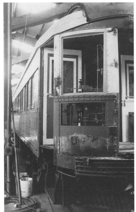
Below: Repairs to the roof and the platform steel framing are well underway in this view of Chicago, Aurora & Elgin interurban 434. JS
