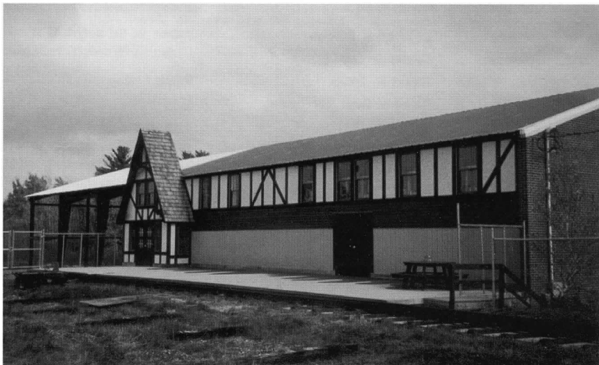
Above: The west frontage of Biddeford Station's building reached the 50 percent completion level in 1997. It will house a restaurant, exhibits, meeting space, and car storage. RD
