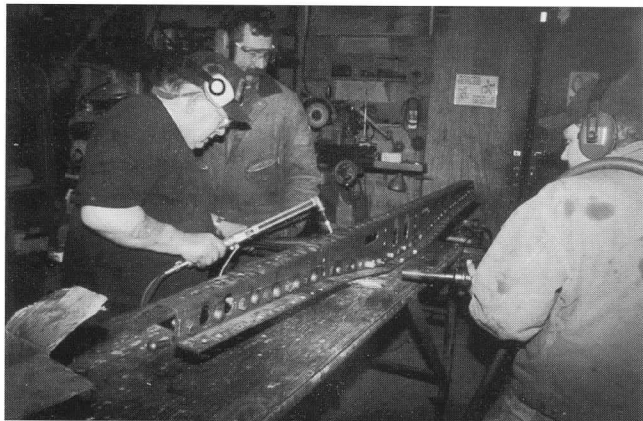
Above: Riveting a body bolster for Rochester 1213: Ed Johnson (left) heats the rivet head, as Gary Jenness (center) holds the rivet with a "buck" for Bill Chapman (right) to drive with the air hammer. DC
