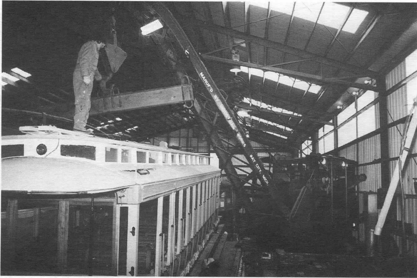
Above: Maneuvering in very tight quarters, staff members Drew Tesseyman (on roof) and Mike Simonds (in crane) prepare to lift Connecticut 303 from its trucks for controller wiring work. DC
