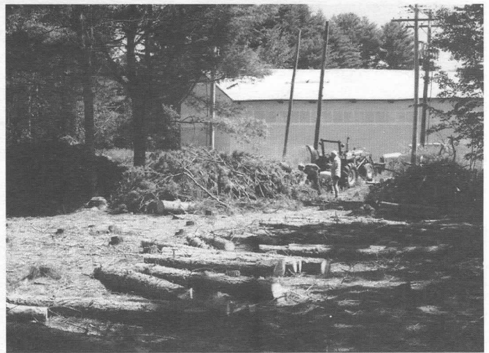
Below: Once surveying was complete, volunteers began clearing the wooded site. The view is toward the back of South Boston Carhouse. DC
