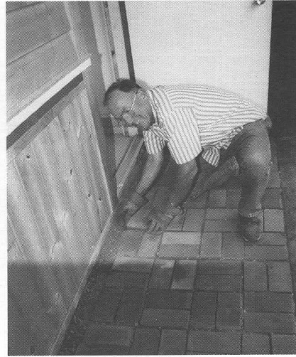
Above: Dan Heffner finishes the new brickwork at the Visitors Center rear entrance. DC
