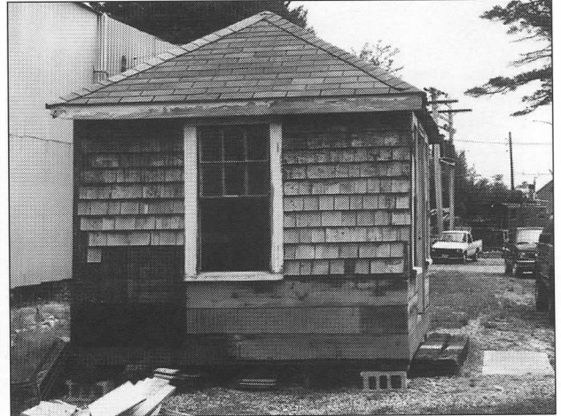
Volunteers are restoring this former Hampton, New Hampshire trolley station for use as a support facility for the adjacent SOAC train. TG
