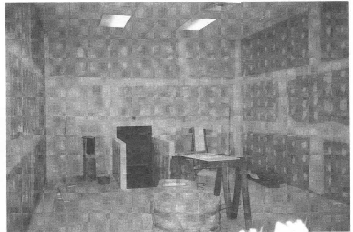
Improvements inside and outside of Biddeford Station were noteworthy in 1993: Above top: The building was extended to its full length with an additional 60 feet of roof and structure. The Great Northern dining car is now completely sheltered. Above lower: A room was finished inside for use by the York County Model Railroad Club which now has ideal conditions for their layouts and operations. RD
