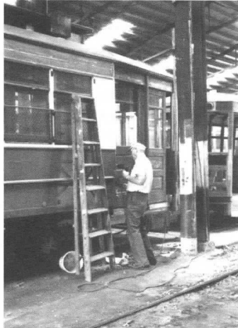
Project Sponsor Dann Chamberlin continues preparations of the exterior surface of Chicago 225 for repainting. JS
