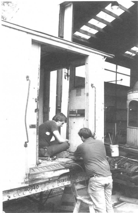
Bill Pollman and Paul Kochs work on the end frame of Boston Orange Line work motor 0521, repairing damage from an accident in Boston some years earlier. When finished, the car will serve not only as an exhibit, but as a useful locomotive for track construction and shifting. JS
