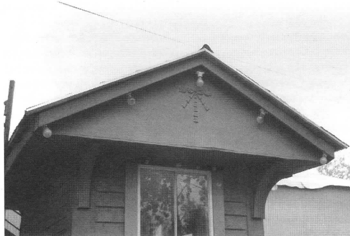
Seashore volunteers made significant progress during the year in rehabilitating this Portland-Lewiston Interurban waiting station for display at Riverside crossing (see photo page 12). This shot shows the roof and window sash complete, and newly rewired lights along the roof line. DC
