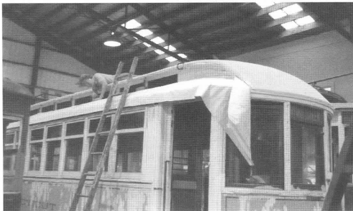
One of the most active projects during the year was the restoration of Connecticut Company 1160. Upper: The car emerges briefly from the Shop as part of a switching operation. Lower: New canvas is applied to the lower part of the roof. JS
