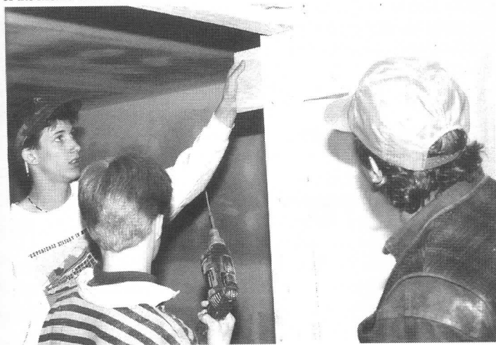
Future Builders Inc. students work on installation of drywall as part of construction of the Moxie Office Suite in the Visitors Center. DC
