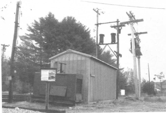
Installed during the year was this new text and photo display explaining the role and history of Seashore's alternating current to direct current power station. JS
