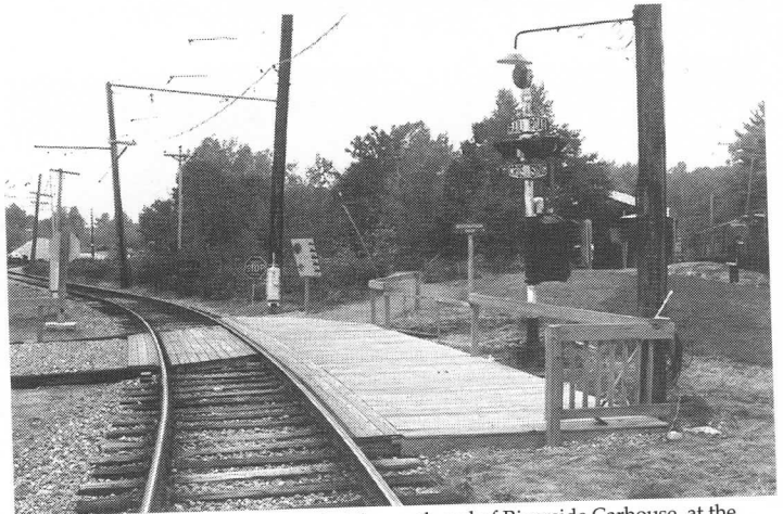
This new platform was constructed at the south end of Riverside Carhouse, at the path leading to the Shop, for use by visitors on the new guided tours and as the future site of the Portland-Lewiston Interurban station undergoing restoration. The path to the Shop was relocated and the area leading to the Shop (at the extreme right edge of the photo) was cleared and landscaped. JS
