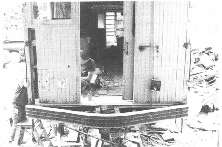
These views show the newly rebuilt end framing from above and below. Seashore volunteers removed all the damaged frame members, fabricated new ones, and installed them. The completed assembly provides a sturdy and rigid structure. JS
