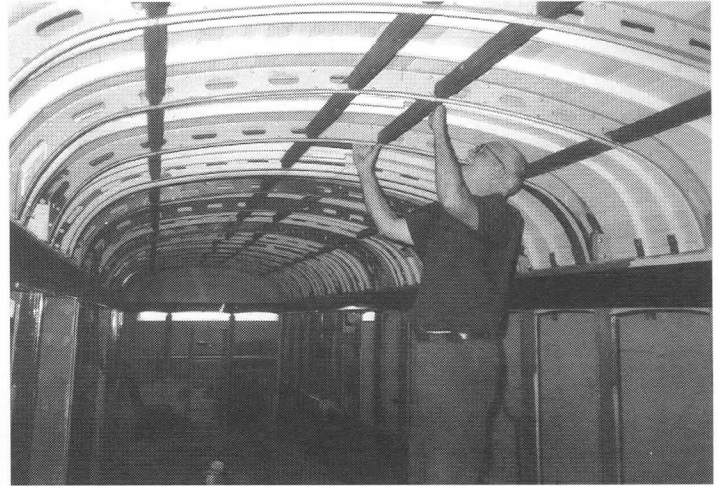
Longtime shop crew member Don Gawthrop adjusts one of the many intricate parts making up the roof structure of Cleveland 1227. The roof sheathing and many finished interior parts were installed during the year. FM
