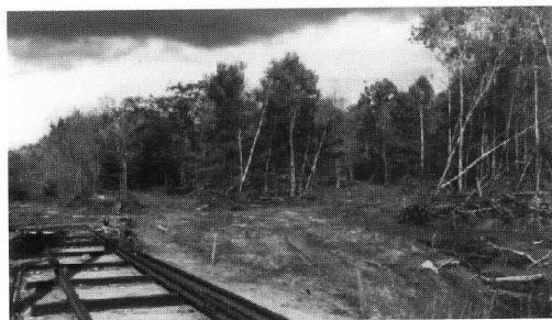
▲ Construction of Talbott Park began in 1991: Upper: The main line reached the park site. Lower: Initial clearing for the loop. J. Schantz
