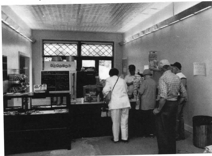
▼ The "Trolley Dog" stand in the Visitors Center progressed in 1991, with newly installed ceiling, wallboard, and lighting, plus improved counters and equipment. D. Black
