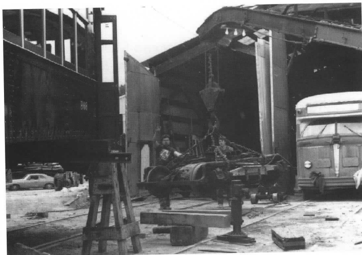
Re-trucking of New Orleans 966 underway in front of the shop. A temporary truck is swung away so the car's own may be rolled under.
