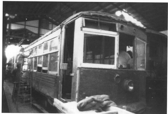
All paint was removed from wood and steel surfaces, and window sash were patched with epoxy, as part of preparation of Sanford, Maine, Birney 82 for service as a display car at the Museum entrance.
