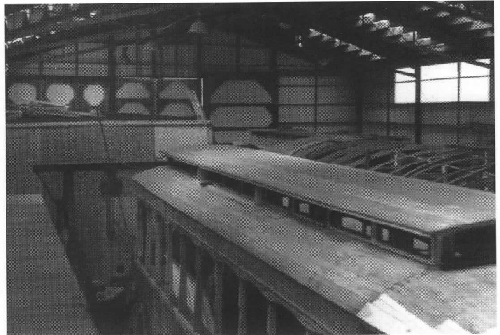
A view from the partially completed visitors gallery shows the insulated box holding Cleveland 1227 (see photos top of page 13). A second box to the right of the one shown has since been added. Bay State 4175 is in the foreground. J. Schantz photos
