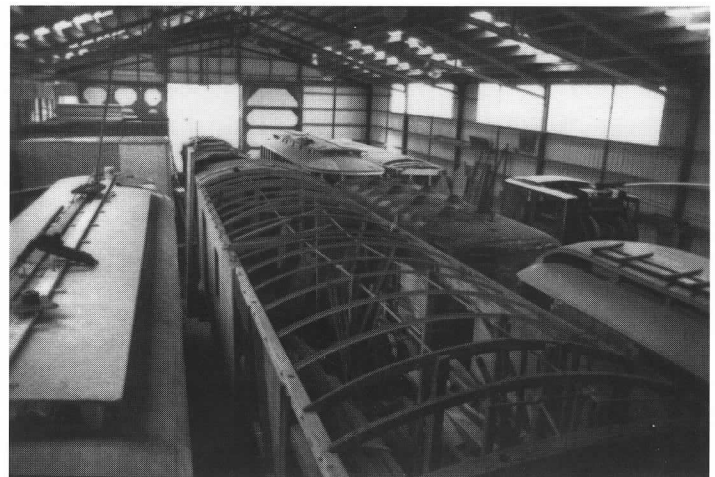
The panoramic vista from the new platform at the end of the Shop visitors gallery (see photo page 16) shows clearly the roof rebuilding underway on Bay State 4175 (at left), Red Line tool car 0553 (center), and Aroostook Valley 70 (right). B. Austin photo
