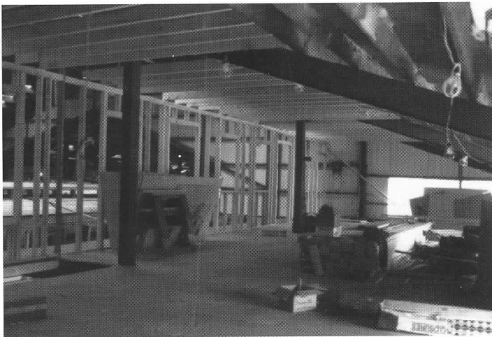
The O'Neil program enabled expanding the second story woodworking area the full length of the building. The new access stairway will be placed in the hole at the extreme left, and the new shop office in the corner to right of center.
