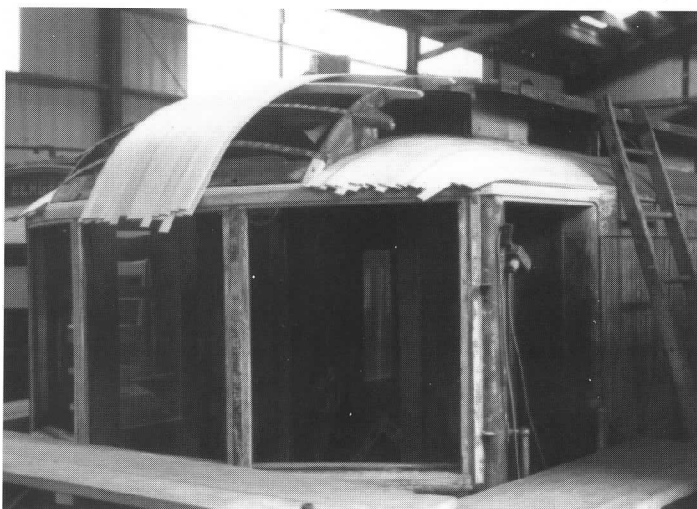
New roof boards have been carefully cut and fitted to the complex clerestory curve of Aroostook Valley 70. A complete roof was installed in 1990. J. Schantz photo
