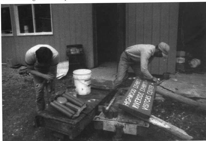
Members work on two different projects outside of Town House Shops. On the left a newly-rebuilt trolley base for Bay State 4175 is primed. To the right a property directional sign receives repairs. B. Austin photo
