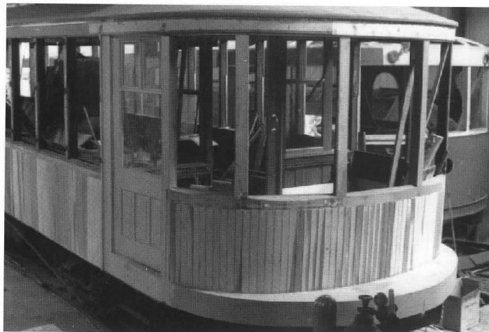
Progress on Twin Cities 1267 in 1990 included fabrication of a new cab door, replacing the folding door that served as an exit later in the car's life. The car also sports new side sheathing and a new massive wooden bumper. D. Anderson photo
