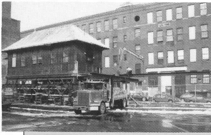
UPPER LEFT: At Albany Street, Payne's crews place housemoving beams under the Station.
