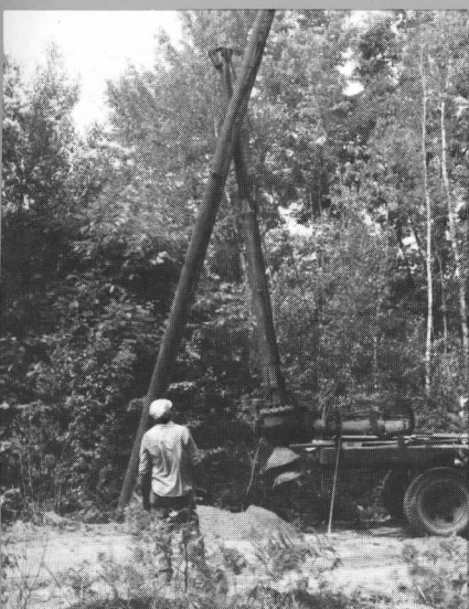
Wooden poles are set on the tangent, steel poles in concrete anchor the wire around the curve. C. PERRY
