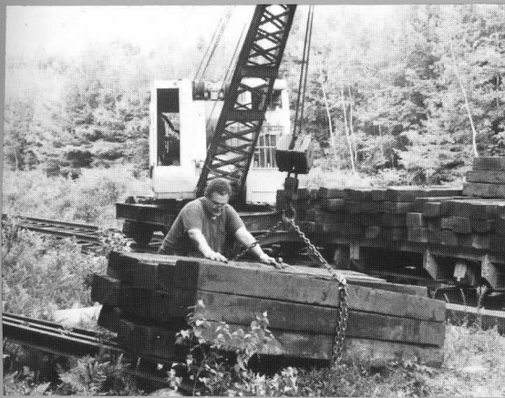
Newly purchased ties are loaded for transport to the extension. D. BLACK
