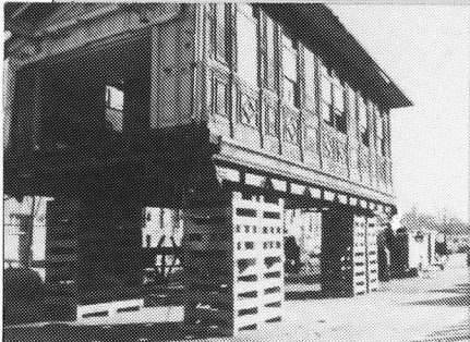
SECOND LEFT: Seashore's crews then carefully cut away the structure for separate transport then reassembly in Maine.
