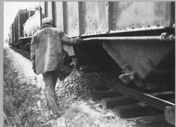
While Seashore's electrified bottom-dump car is on lease to the MBTA, a railroad hopper car is used to spread ballast. JDS
