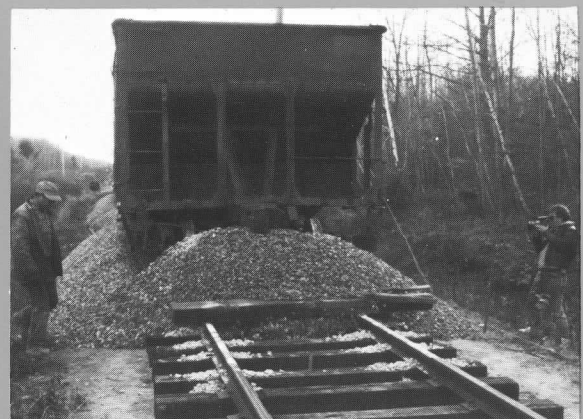
As the hopper lacks the fine adjustments of the bottom-dump car, ballast must be leveled by means of ties pushed in front of the wheels. JDS
