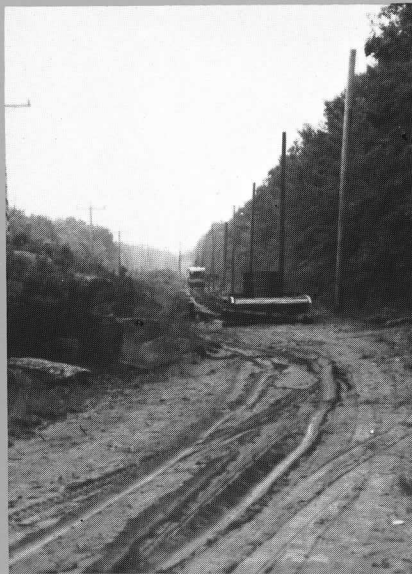
ABOVE: Poles and rail reach the end of the tangent. D. BLACK
