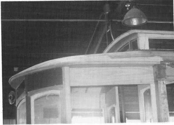
LEFT: The careful craftsmanship used to fit new roof and vestibule pieces on Bay State No. 4175 is evident in this view. Final roof canvas is the next step. D. BLACK
