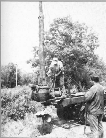
Before track is laid, holes are bored for line poles. D. BLACK
