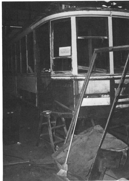
LEFT: The latter day step well and door assembly are removed and framing is being rebuilt to bring Twin Cities 1267 back to the configuration shown on the rear cover. JDS
