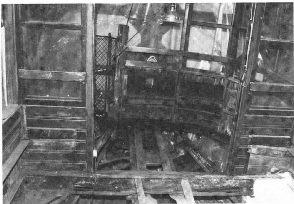
Before and after views of the rear platform of Twin-Cities 1267. Extensive replacement of corroded frame members was necessary. Subsequently the rear platform upper framing has been rebuilt. JDS
