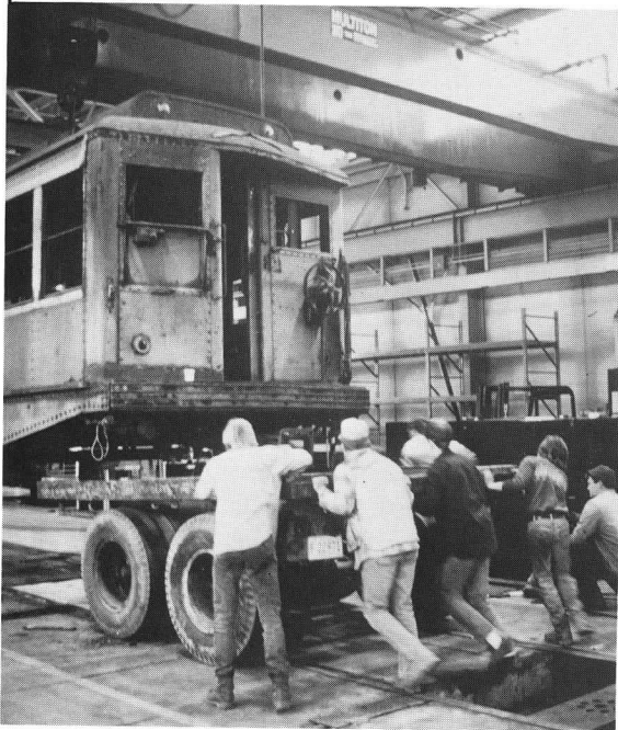
Another view of preparations to move 0753 at the Cabot Shop of Boston's MBTA. Volunteers move a dolly under the end of the car as it is hoisted by an overhead crane.
