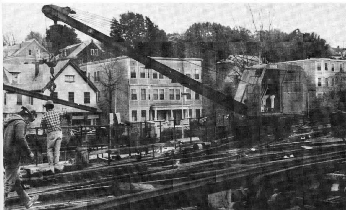
Their crews manned the Burro, which was used to move parts within reach of the larger crane below. TSdeB
