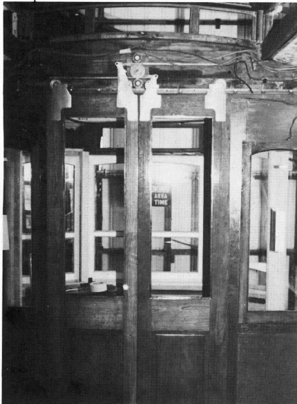
Completed bulkhead doors have been hung and match nicely the all new bulkhead partitions constructed for Eastern Mass. 4175. The sliding hardware mechanism at the top of the doors was donated by the Gomaco Company of Ida Grove, Iowa. TSdeB
