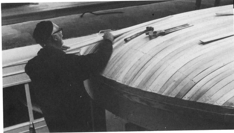
The most intricate step in rebuilding a roof is determining the taper for the last few roof boards to curve over the ribs. Here Don Gawthrop, a professional with the Department of Street Railways in Detroit before coming to Seashore, measures the last few pieces for New Orleans 966. TSdeB
