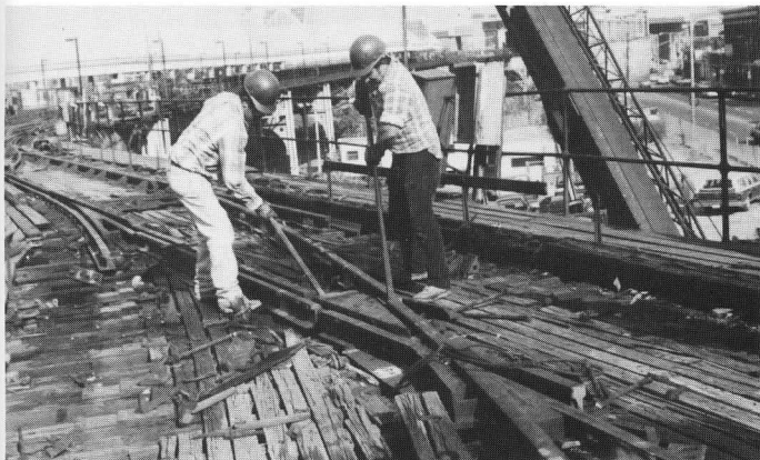
White's crews painstakingly unbolted all components, which otherwise would have been demolished quickly. TSdeB
