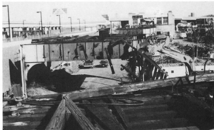
Once the track was gone, giant hydraulic shears made short work of the structure. TSdeB
