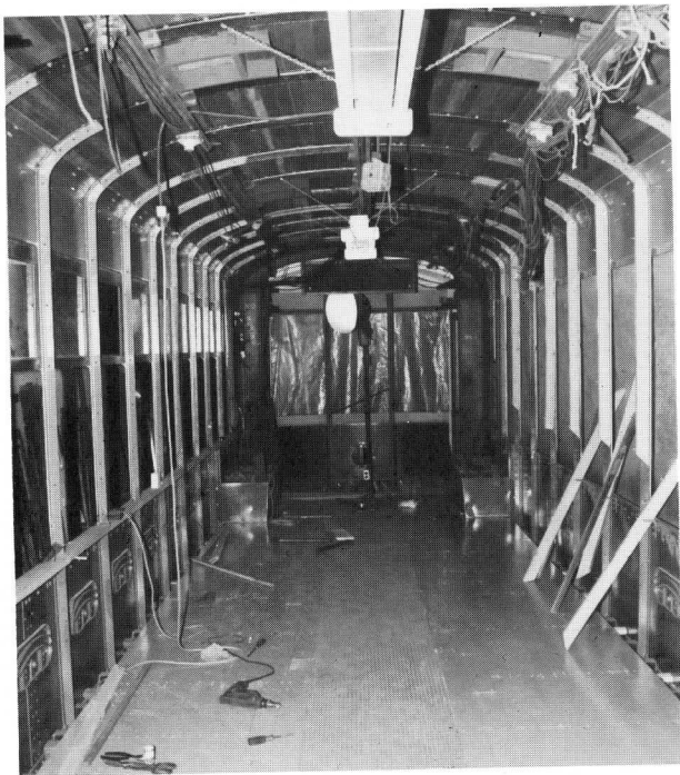
This interior view of 966 shows the new floor and roof, the rebuilt steel sideposts, plus the first new sash and window sill pieces. JDS
