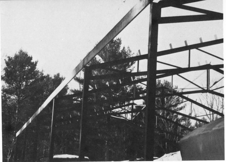
Museum volunteer crews have erected steel columns and trusses at the rear of Fairview Barn in this shot. Framing and exterior sheet remains to be applied. FRED PERRY
