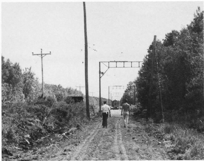
Before tracklaying could begin in earnest, the roadbed below and above Tower 8 was in need of extensive drainage and ditching work. It was considered more expeditious to remove completely 300' of track to accomplish this work. WOOLNOUGH
