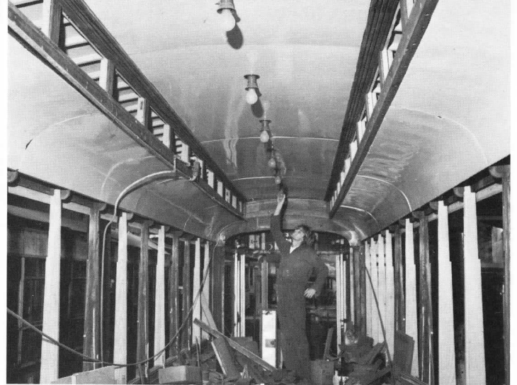
With new steelwork supporting the once drooping vestibules, work could be concentrated on rebuilding the car's interior. Headlining, as shown in photo, had been restored as part of 1984's work. WOOLNOUGH
