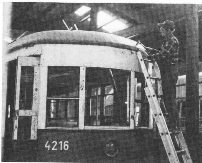
With most of the transportation costs of moving Vienna 4216 (formerly Manhattan/Bronx Third Ave. Rwy. 631) having been raised through donations to the President's Club, attention has now been turned toward its restoration. Here repairs to the roof bonnet are underway. TSdeB
