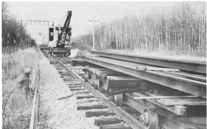
ABOVE — The Swenson Quarry rail is moved out for the main line extension on small flat cars with the assistance of the now indispensable Burro crane.
