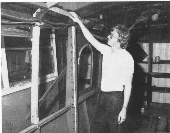
Work has been accelerated on Wheeling Curveside No. 39. One of car's major sponsors is shown fitting a backing strip into roof framework in preparation for application of wood roof sheathing. WOOLNOUGH
