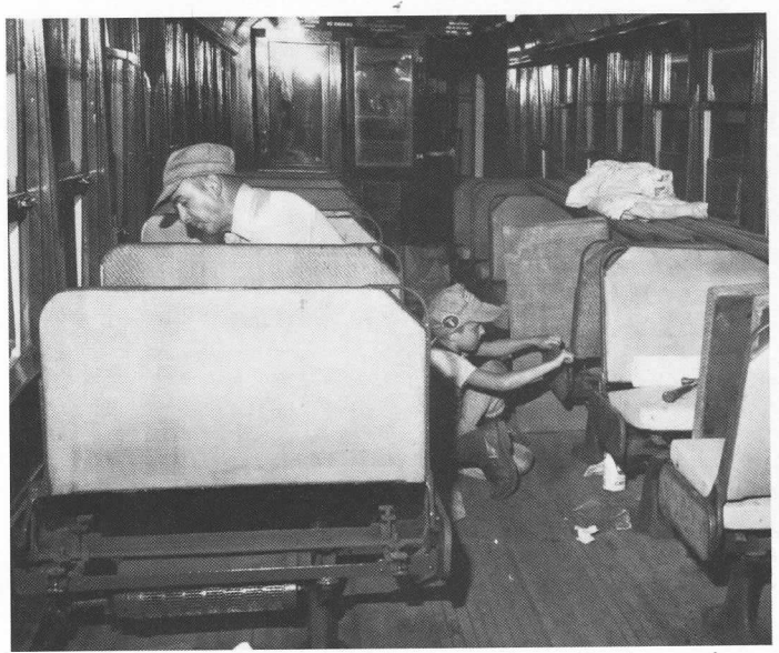
A father and son team has been doing extensive restoration work on Chicago Surface Lines 225 for some time. Here, they are working on 225's interior finish. WOOLNOUGH
