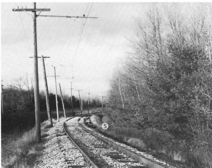
The rail changeout program progresses steadily northward as the worn Atlantic Shore 70 pound rail is replaced with A.S.C.E. 85 pound rail. Re-alignment of the curve and rebalasting with crushed stone are included in this program. R. T. Lane
