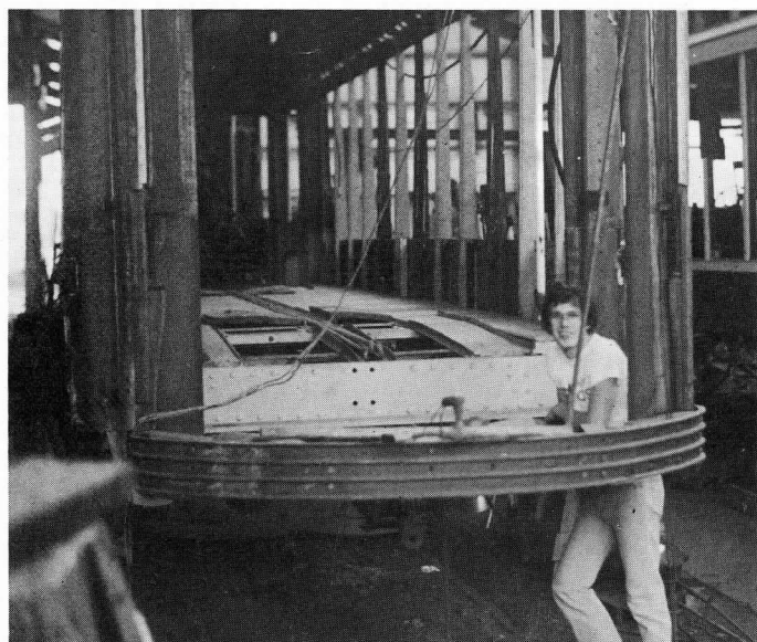
ABOVE — 4387's platform with major steelwork replaced in readiness for reconstruction of "north" vestibule in '83 T.S.de B.
