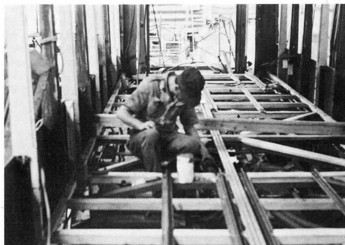
ABOVE — Shop Foreman, Donald Curry painstakingly installing wood furring to provide level floor. T.S.de B.
