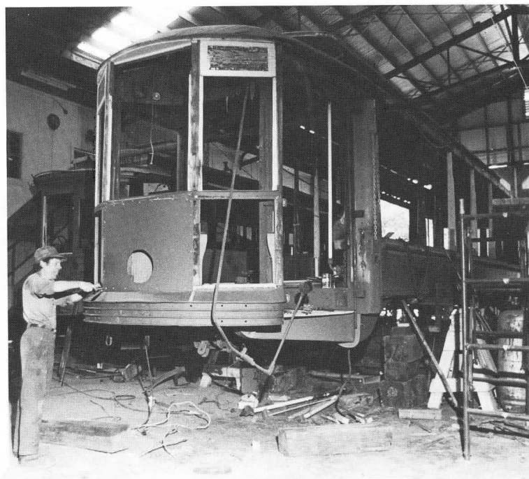
One of the several more difficult jobs in the rebuilding of 4387's vestibules was the fabrication of the new platform knees — not only of a novel design but originally shaped by an air hammer at the Laconia carbuilding works, while the replacements had to be custom made by a Society member virtually by hand. Once these were in place the first vestibule began to shape up rapidly under the watchful eye of the Shop superintendent.
