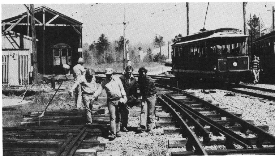
The decision many years ago to extend Riverside Barn one additional bay at a time when inside storage space was so much in demand created a problem long left unresolved. The switch on a curve providing the two lead tracks into the barn on the south side would have to be relocated eventually in order to permit closing in and installing doors at this end of the Barn. 1980 proved to be the year. The view at the left with car No. 31 passing by on the Main Line shows the track crew dismantling the old layout.
