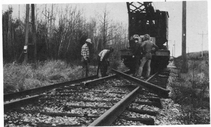
In the fall a rail cropping program was carried out on the "Tower" Section of the Main Line. Crane car #3246 assists. Another year such work may be turned over to the recently donated Burro Crane with its longer reach. — Woolnough —
