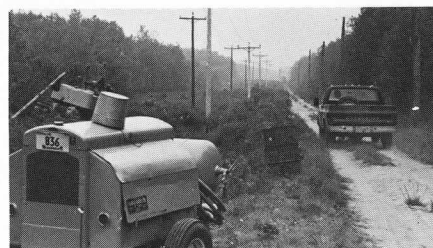
This telephoto view down the right of way shows the new poles of the Central Maine Power Company before the wires were moved over and a streetcar at the present end of the main track. Woolnough Photo
