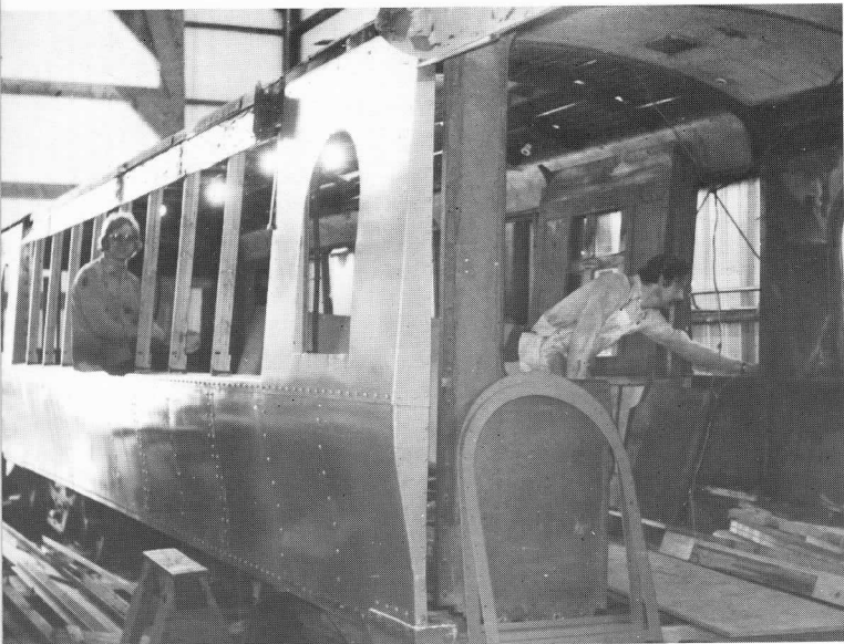
New window posts being installed in Cincinnati curve side. Car's Sponsor framed by center window. — Lane
