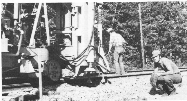
McWilliams Multi-Purpose Tamper putting finishing touches on main line curve leading out of M. & S. C. Jet — Lane.
