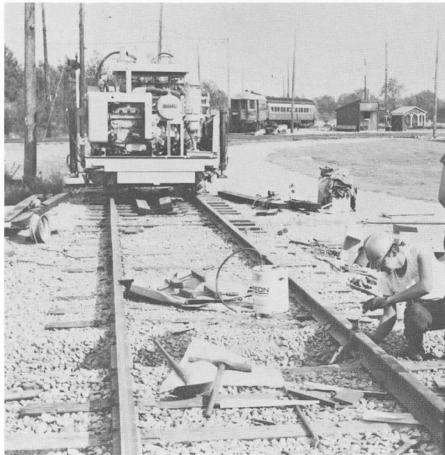
Two views of the Butler Grove Lead Track during its reconstruction. Below/left, the partially built turnout looking south at railhead level. Above, finishing touches are made to a thermite welded joint. Brillante and Lane photos.
