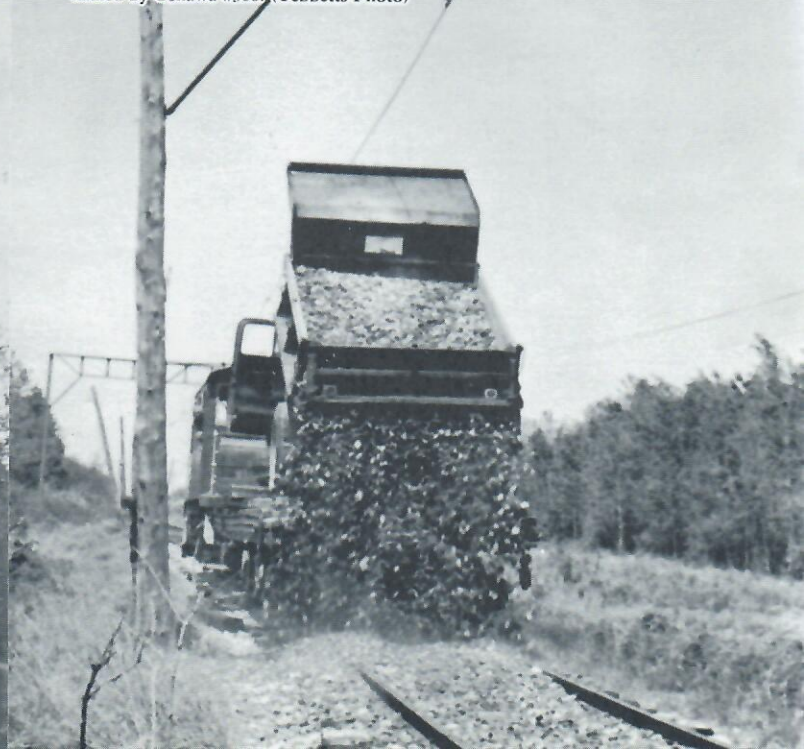
Main line ballasting underway during the fall of '72. Dump truck on flat car hauled by Oshawa #300. (Tebbetts Photo)
