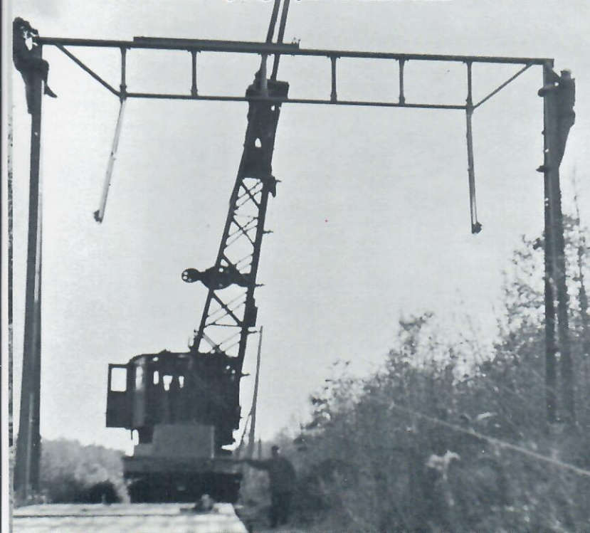
Tower 8 erected at end of the year, completing current extension northward. Crane Car #3246 setting bridge in place. (T. Santarelli Photo)
