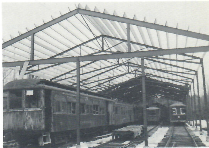
Trusses in place, roof purlins fastened in position, ready for 22' roof sheets. (Tibbetts Photo)
