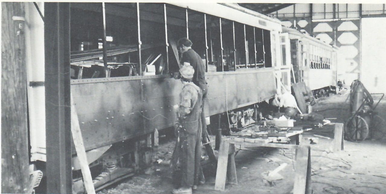
A new skill acquired by Seashore shop force. New steel plates hot-riveted to frame of Montreal 2052. A very useful skill for future use in restoring other cars. Tom Murray at work, Don Curry supervising. (Tibbets Photo)
