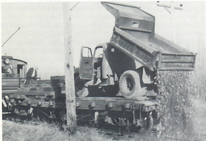
Ballasting the outer 1200' of the main line utilizing Oshawa 300, bar flat car and the dump truck. Photo by Jim Tibbetts
