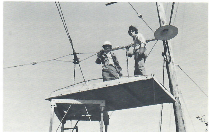
Positioning new frog into overhead. Paul White and John Williams at work with Line Car S-71. One of many upgrading projects undertaken by the Line Department during 1971. (R. T. Lane Photo)
