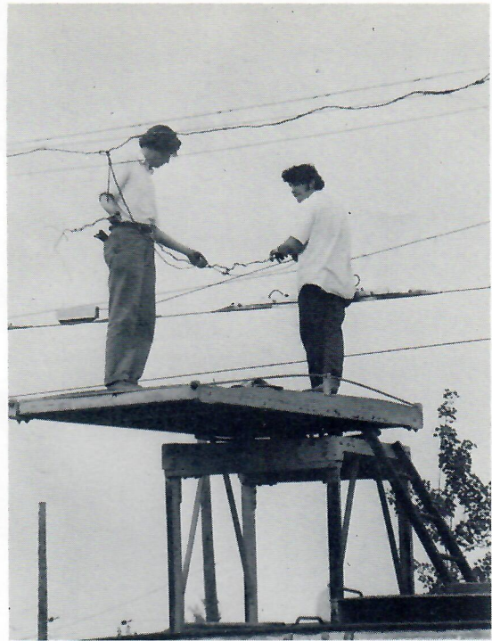
Paul White supervises installation of Cheatham track switch contactor from roof of S-71. Photo James E. Tebbetts
