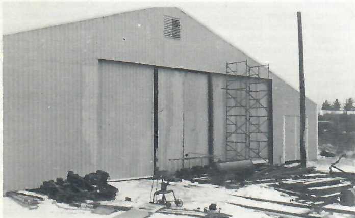
North end of new car shop now completely closed in. Photo by James E. Tebbets
