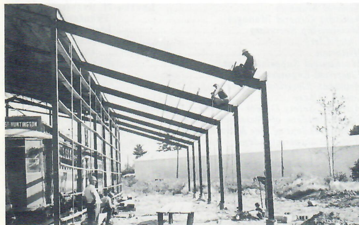
#3 shows roof purlins being fastened in place over lean-to being added to shop where machinery will be housed. (Lennon photo)
