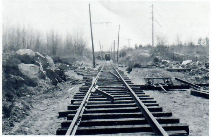
Looking South to Syracuse station — siding to be put in for hauling out fill. (John Coughlin photo)
