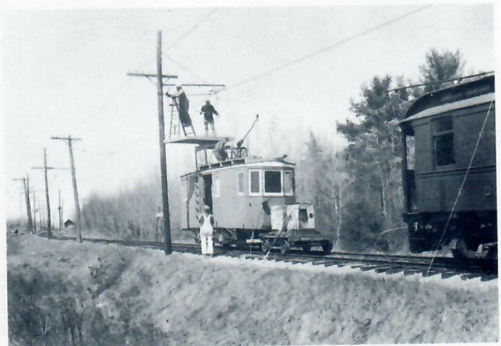
Line crew with ex Eastern Mass St. Ry tower car converting last of consolidation section to catenary. Ex Atlantic shore 108 in right foreground. (John Coughlin photo)
