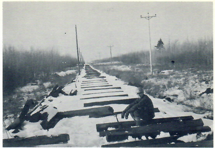
Looking ahead into the coming year track materials are stretched out as far as the eye can see. Project Engineer and Trustee Tolbert McKay pauses momentarily while lining ties for the Main Line extension, which is being carried out under his supervision. (photo by John Coughlin)
