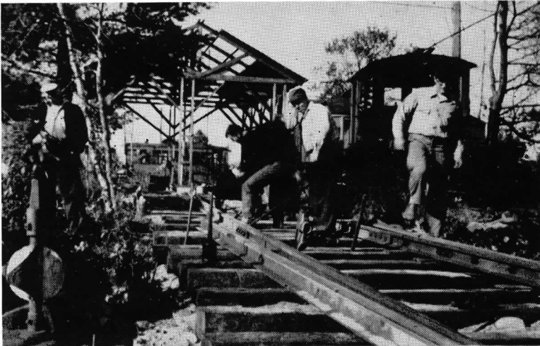
CREW LAYING TRACK into new shop which is seen under construction in the background. Cars 100 and 108 appear at right.
