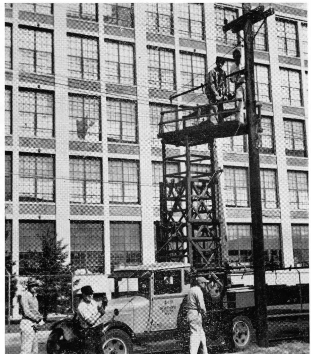
NO. S-117 and the Seashore line crew in Sanford salvaging trolley brackets.
