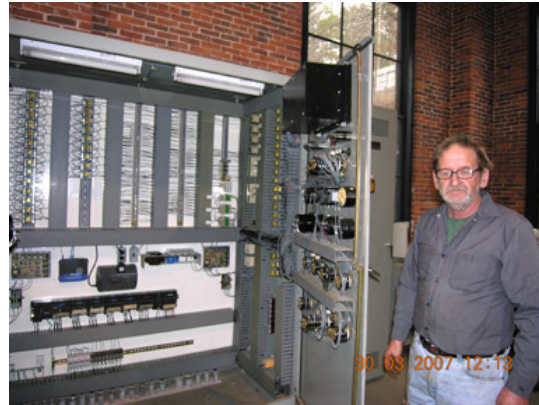
Iain Taylor showing the new generator controls.
