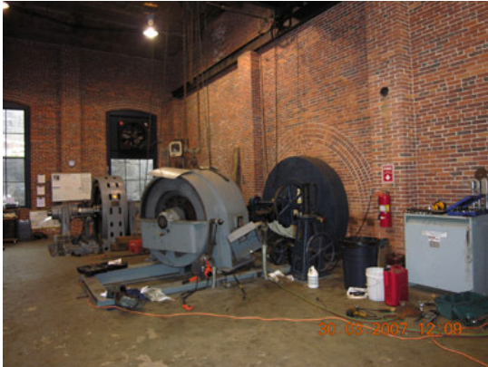
The 1960s era Westinghouse generator.
