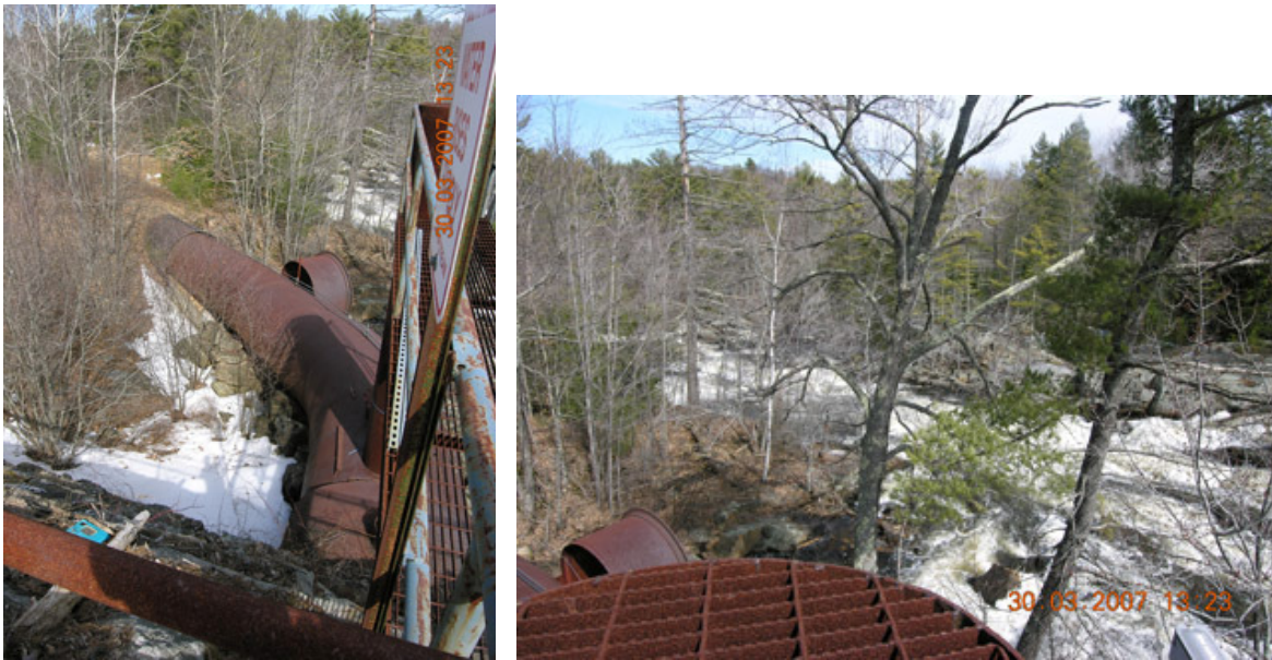
The penstock leading to the power station. The Mousam River. Note the discarded penstock gate and the remains of the snow.
